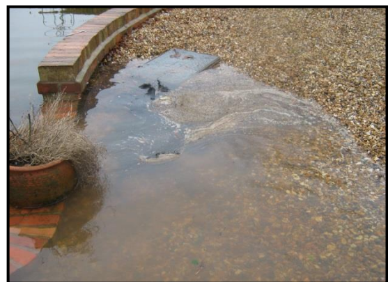
A blocked land drain forcing water to escape through an inspection chamber
